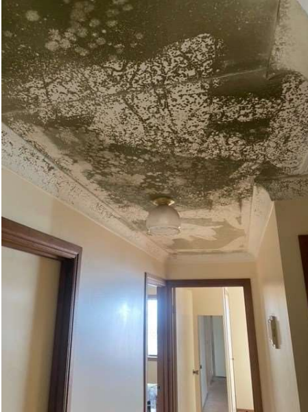
Ceiling Mould – 173 North Street, Toowoomba
